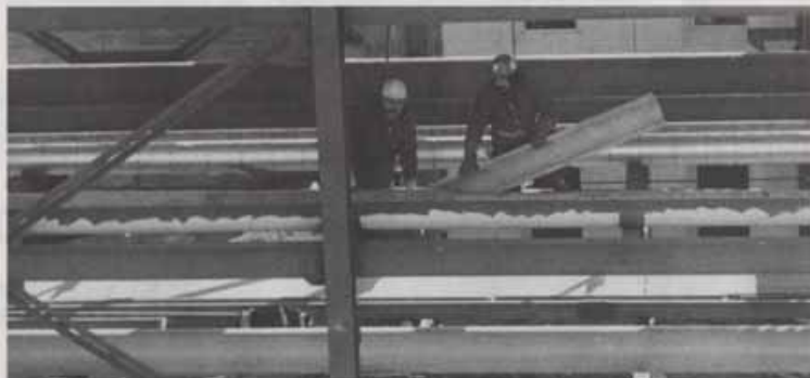
Workers atop pipe racks at the Norsk Hydro plant install extended-length 3-metre pipe insulation.
