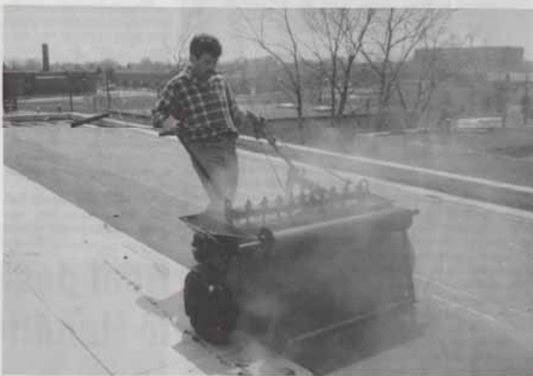
Trio Roofing crewman spreads asphalt over Perma-Therm boards during the product's field testing.
